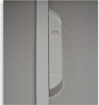
> BE-BOX-24 with extension plastic covers installed along a wire way
